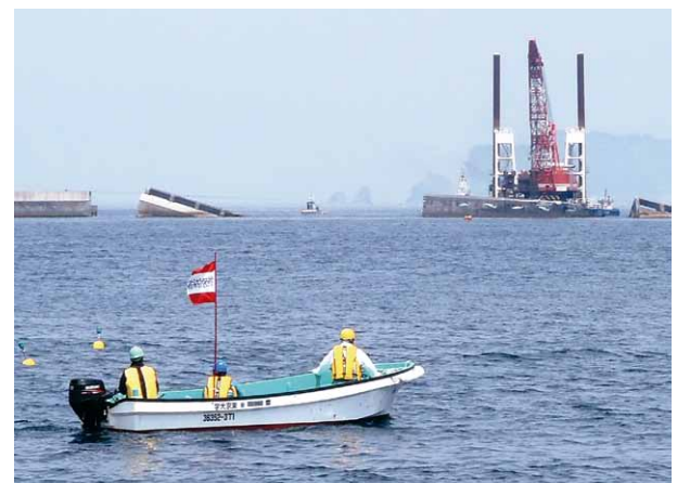
東日本大震災で破壊された釜石湾港防波堤付近での海洋環境調査 Observation of the marine environment in Kamaishi Bay, damaged by the Great East Japan Earthquake
